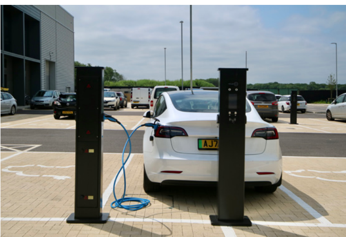
Fig. 175 - EV charging points to all buildings
